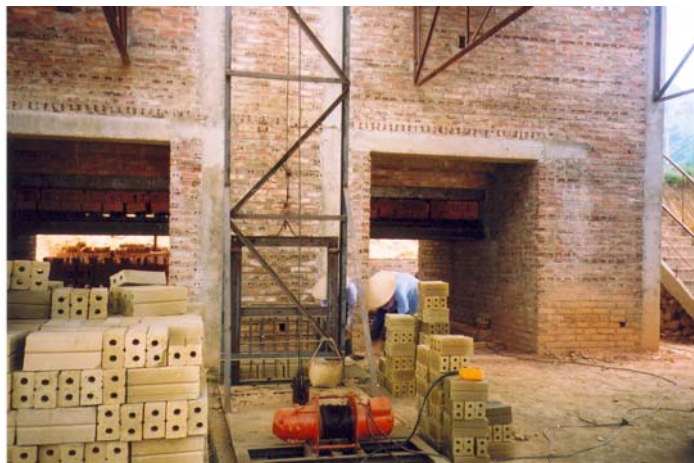
Winch for lifting
